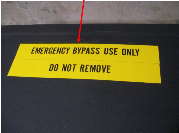
Figure 2 Location of Emergency Hypo Hose
