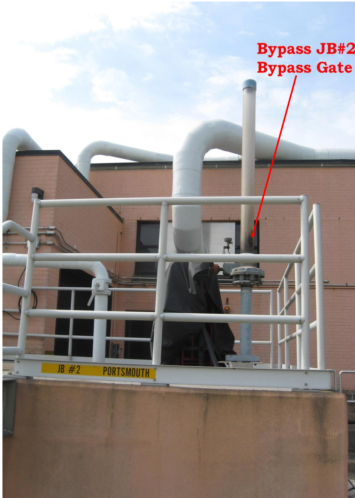
Figure 8 Bypass Gate #2 at JB # 2
