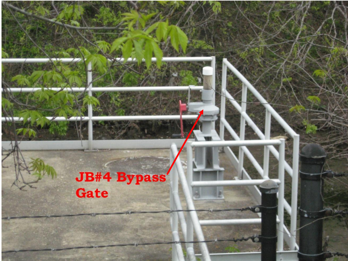
Figure 9 Bypass Gate # 4 at JB #4
